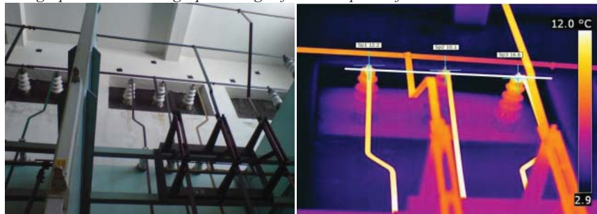
Picture 2. Photographic and thermographic image of internal parts of conductive insulators on a 35 [kV] side
